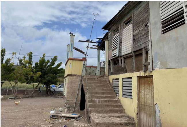
Wanda’s two-story house has been designated unlivable. (GSR photo / Soli Salgado)
