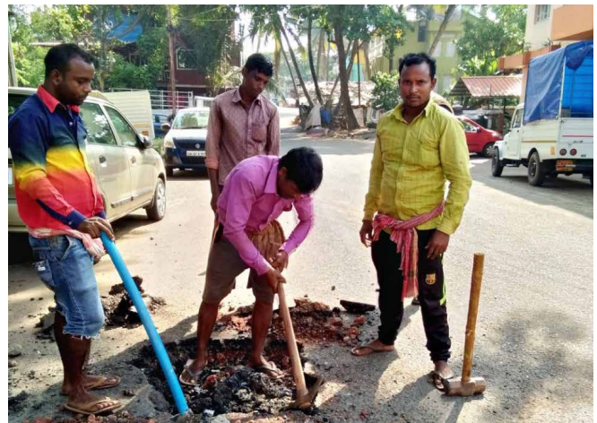
Migrant men repair a road in Mala, a village in Goa, western India. (Lissy Maruthanakuzhy)
