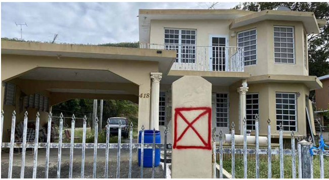
Even if a home appears not to be damaged superficially, structural engineers may find integral damage that make it dangerous to go inside. They designate a home either red or green to differentiate. (GSR photo / Soli Salgado)
