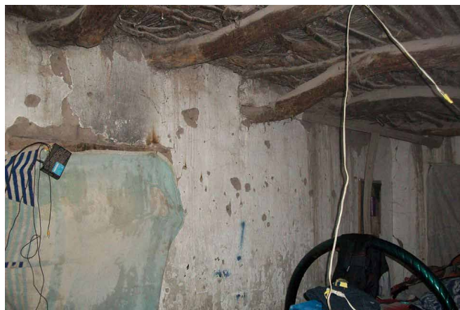
Rafa's home, in Villa García, Zacatecas, Mexico, contains a room that had to be removed. It was attached to the kitchen and another room that fell down. It was being used for one of the adult men in the family, and snakes were living in the ceiling. (Frances Smith)
